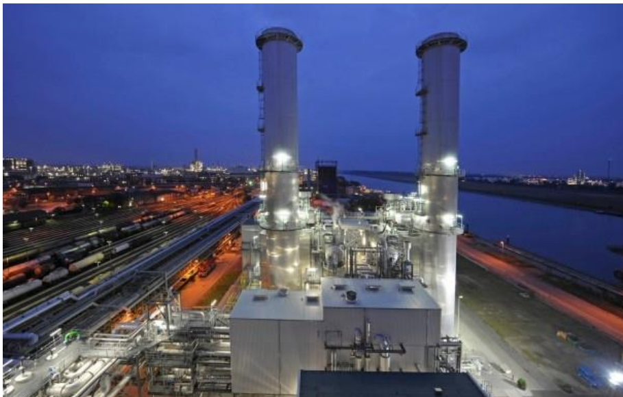
This power plant at BASF's Ludwigshafen site generates electricity and heat for the production facilities with very high efficiency. (Photo: BASF SE)
